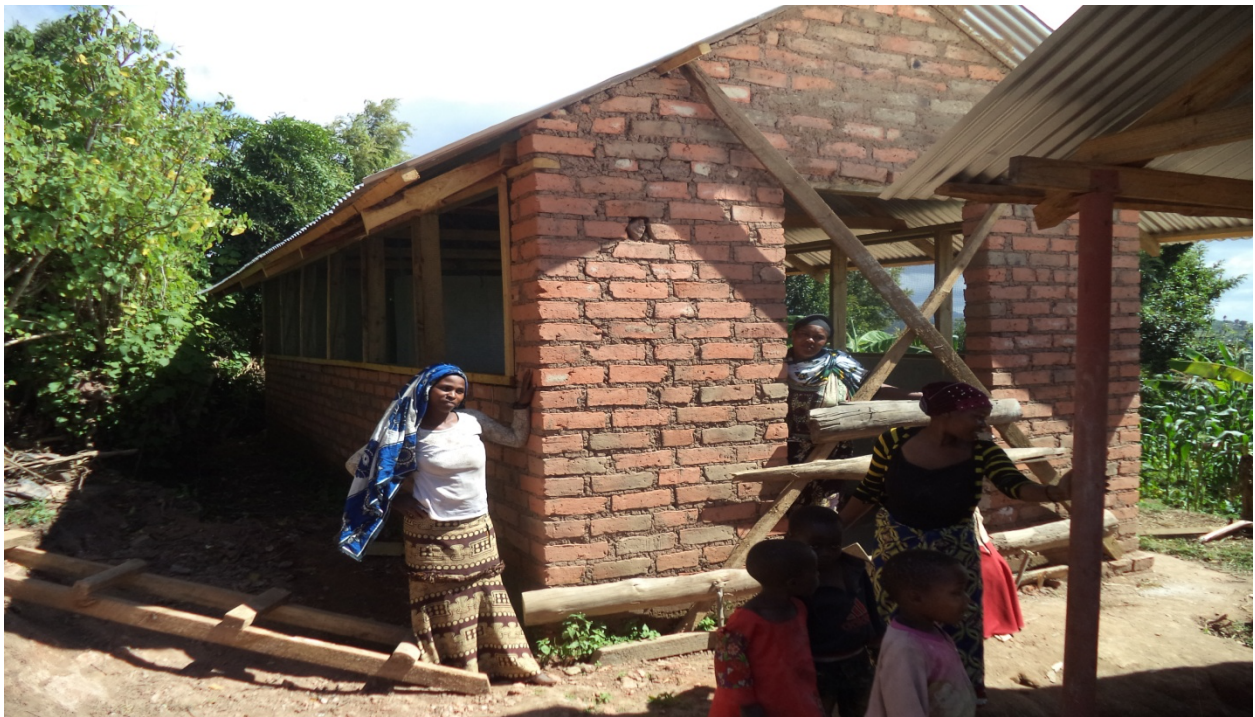
Photo 1: Training building of Kwekishasha Pottery Group looking in a finishing construction stage (Front view).
